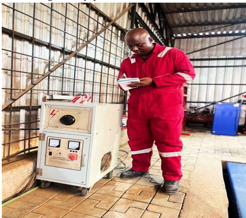
Figure 5. Battery Charging Machine at Nut and Bolt Jahi, Abuja, Nigeria
